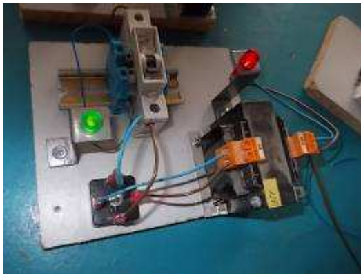
Photo 39: Being from out of Switzerland some small transformers 230 volts, 24 volts, and have to buy in the market as a rectifier for 1 franc.
