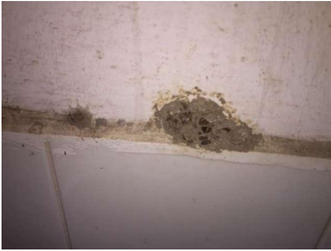
Wasp nests in the toilet. Location: WC behind the space 6. Photo WS10_320
