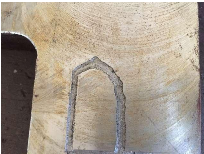
The care during milling is important. What is failed to be re-welded shut and re-made. This is better than to be like that. It's a shame, so throw a vice. But it has to be thrown away before they see Third, if this is not fixed! Room 2 Photo WS10_120.
