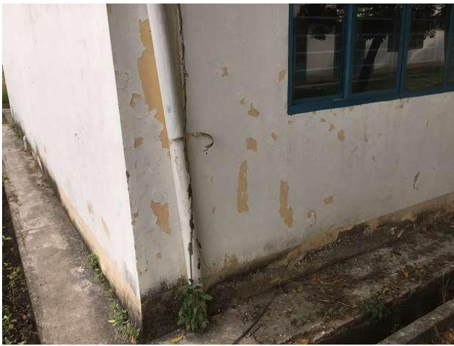
The entire facade of the school were repainted about 3 years ago. The costs we have halved the school. Why see in Vietnam building shortly again like that? Is it the quality of work? Or the material? Location: Exterior space 3b. Photo WS10_330
