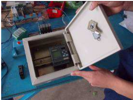
Photo 10: In the space 6a in the electronics department, we are now beginning the so-called "tropical Cabinet Control" boxes. We want to make a monitoring against condensation in electrical cabinets. The goods we bought. However, we will send everything to Switzerland and there make ready. Here in Vietnam, we still recognize much too little on quality.
