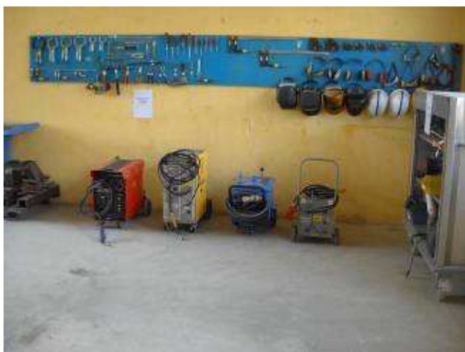
P24: Welding area, two system gas and two electrode welding up to ..... Amp.
